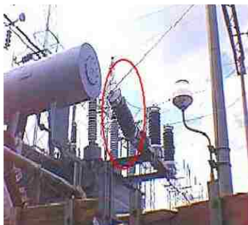
(a) Broken Bushing of a Transformer
