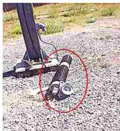
(b) Broken Bushing of a lightning rod
